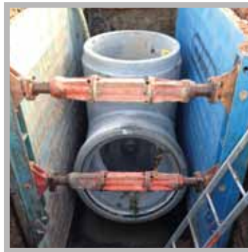
1200mm end entry manhole complete with hydrobrake
