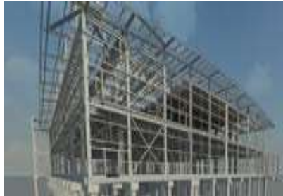
SatGate, Lithuania Full structural design for a new greenfield, two storey DC, including a hybrid precast concrete shell and steel frame together in a barrel vaulted roof.
