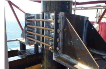
Structural Modifications to High Pressure Vent As part of the interfacing of drilling rig (EnSCO 122) with nodal gas platform (K14-FA-1) in the Dutch sector of the Southern North Sea, Pinnacle designed an interface for a 27m personnel gangway between the drilling rig and the production platform along with significant works to re-route the main platform high pressure gas vent.
