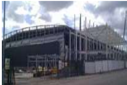
Equinix Group, London Structural modifications and fit out works over 3 phases. Complex steelwork support design for critical services utilising BIM and cloud point surveys.
