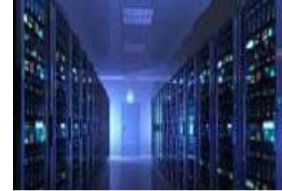
AMS, Phases 1-4 Amsterdam Four separate building projects over 3 year period, 10-15MW whitespace each, providing detailed structural and civil packages for conversion of existing warehousing into new colocation space including new mezzanine levels.
